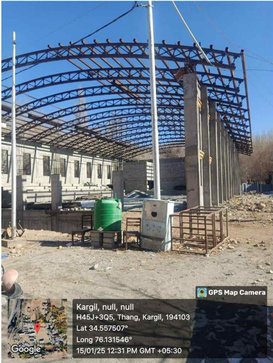
4. Indoor Stadium, Gym and Multipurpose Hall for the Department of Physical sciences
